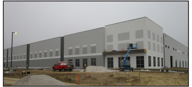
Scannell Properties | West Chicago, IL DuPage Business Center | 250,000 SF Summer 2020 - Estimated Completion
